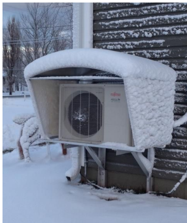
FIGURE 3 HEAT PUMP MOUNTED ON SIDE OF BUILDING
