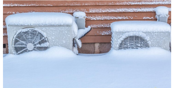
FIGURE 2 HEAT PUMP BURIED IN SNOW
