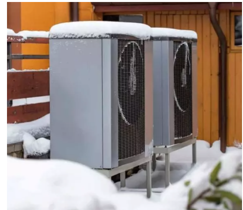
FIGURE 4 HEAT PUMP ON STAND
